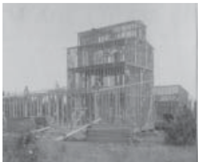
Construction of the first Martin Mill, 1913. The wood structure burned several years later. Photo courtesy of Cheney Historical Museum.
